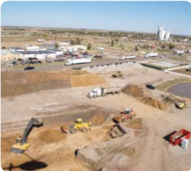
Top: The groundbreaking for the new Kiowa County Memorial Hospital was held in October 2008, more than a year after a tornado wiped out the old facility. Bottom: Construction crews prepare the new hospital site in Greensburg, Kan., with temporary facilities visible in the background.
